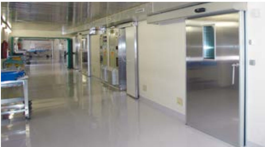
Corridor of the operating ward with PSE stainless steel doors with 45° barter suitable for cleaning
